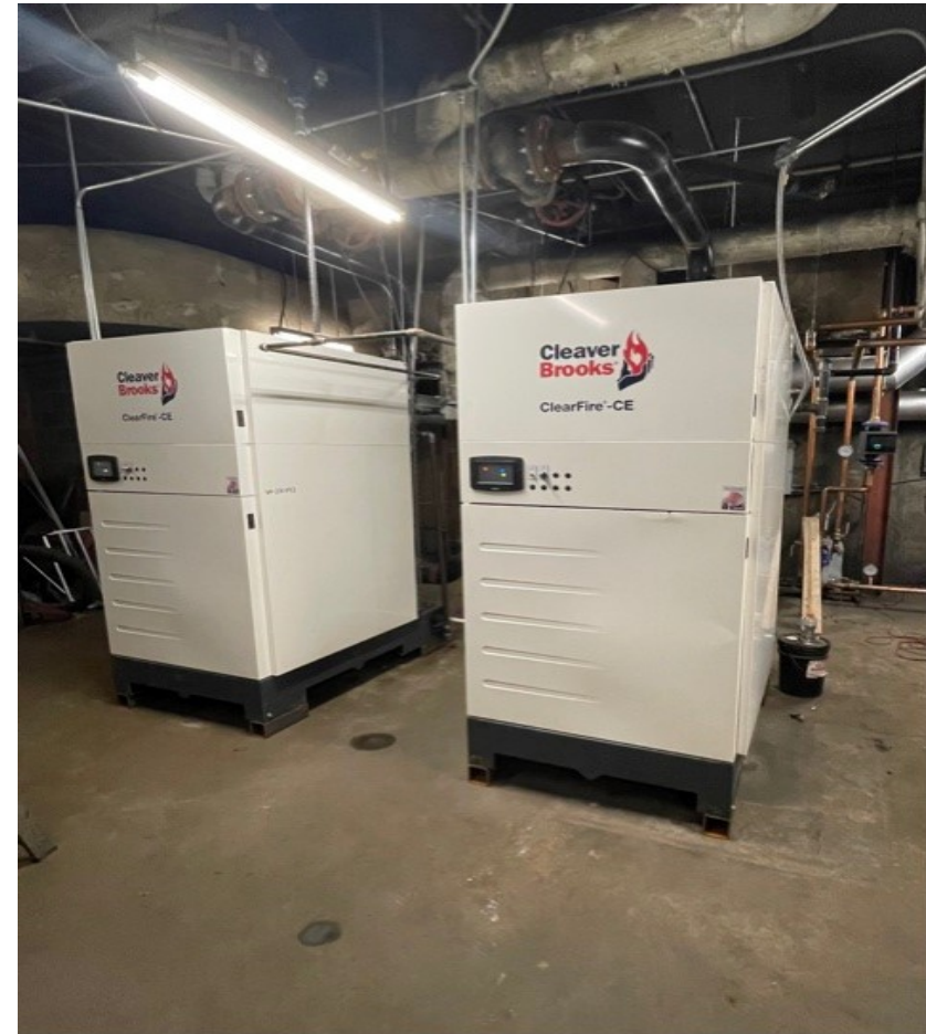
In with the new LP Gas Boiler
